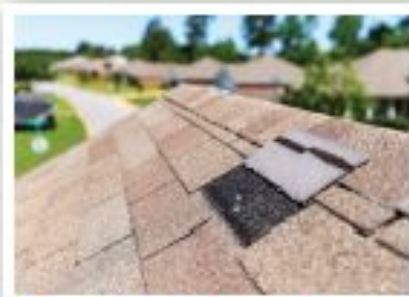
A storm occurs in your neighborhood leaving behind unseen damage.
