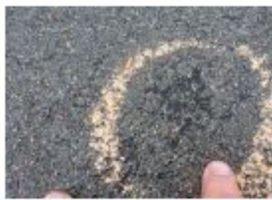
Our trained professionals will perform an inspection to check for damage.
