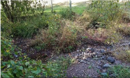
View upstream where the creek bed is quite full of silt, rock, and vegetation. This is part of the problem.
